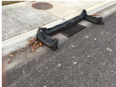
Stops Dirt & Covers Curb Cutout
